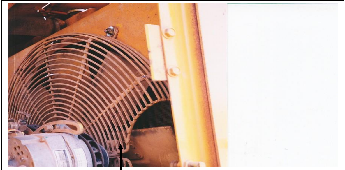
Fan screen rotated 90o so joint is horizontal
